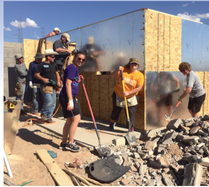
The team began with only a concrete slab, and by the end of the week Mariana was able to move into her new home.
